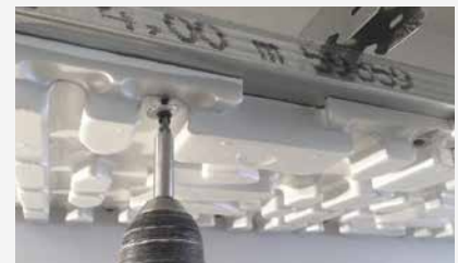
Installation and fitting of head panels on the metal support structure with 35 mm screws
