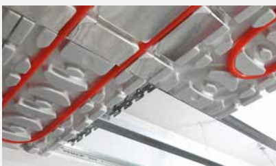
Installation and fitting of R883-1 panels and pipes along the preformed panel and head housings
